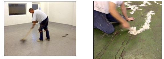
Pic 2. Sweep the floor, remove any highpoints and patch repair or level any cracks or low points.
